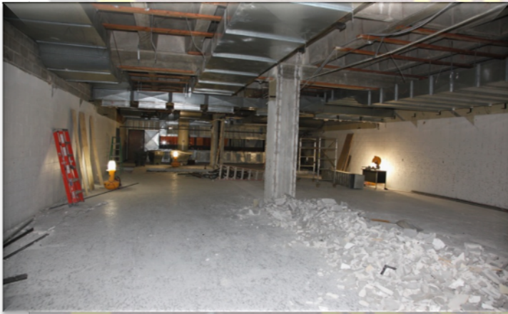
Central's old gun range during demolition work for the installation of a high-density evidence and property storage unit
